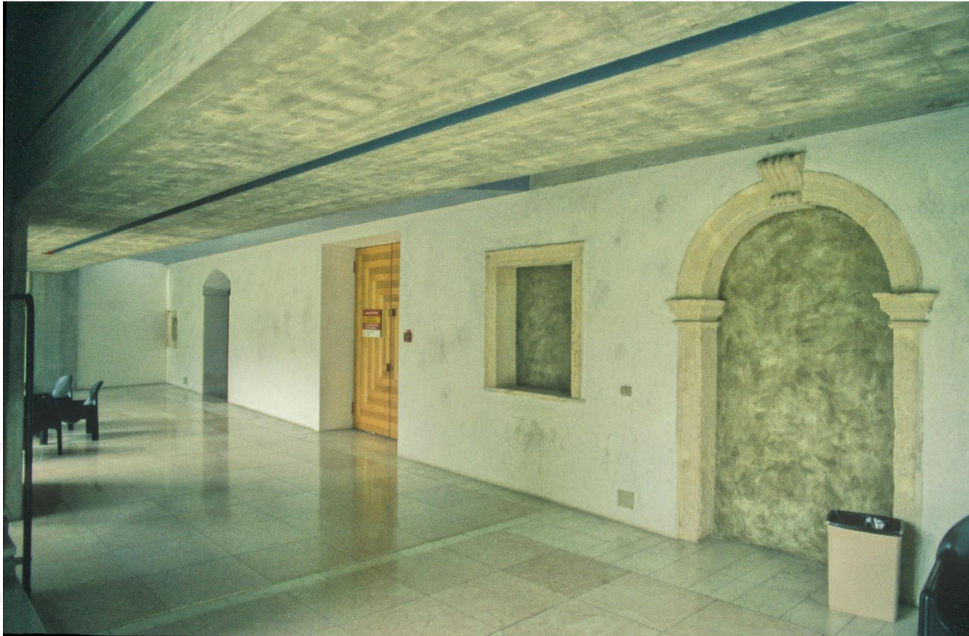
An improper addition in a preexistence Villa (CB 1986)
